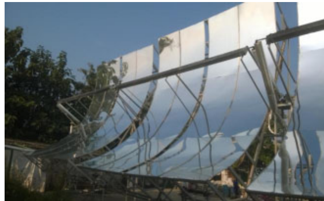
Parabolic Trough Collectors at Siddhartha Surgical, Vadodara (263 m 2 ; Process Heating)
