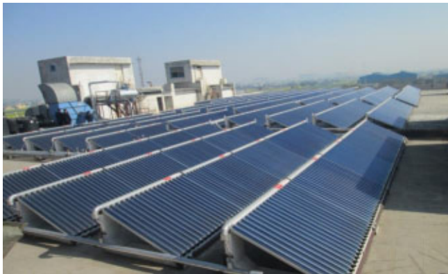
Non- imaging Collectors at Neel Metal, Gurgaon (612 m 2 ; Process Heating)
