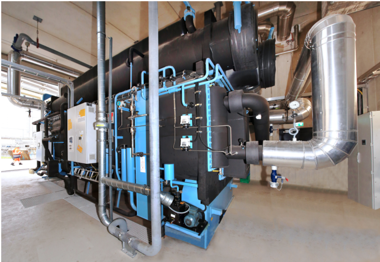
Figure 11: Implementation of the new absorption heat pump, Source: Klimafonds / Krobath
