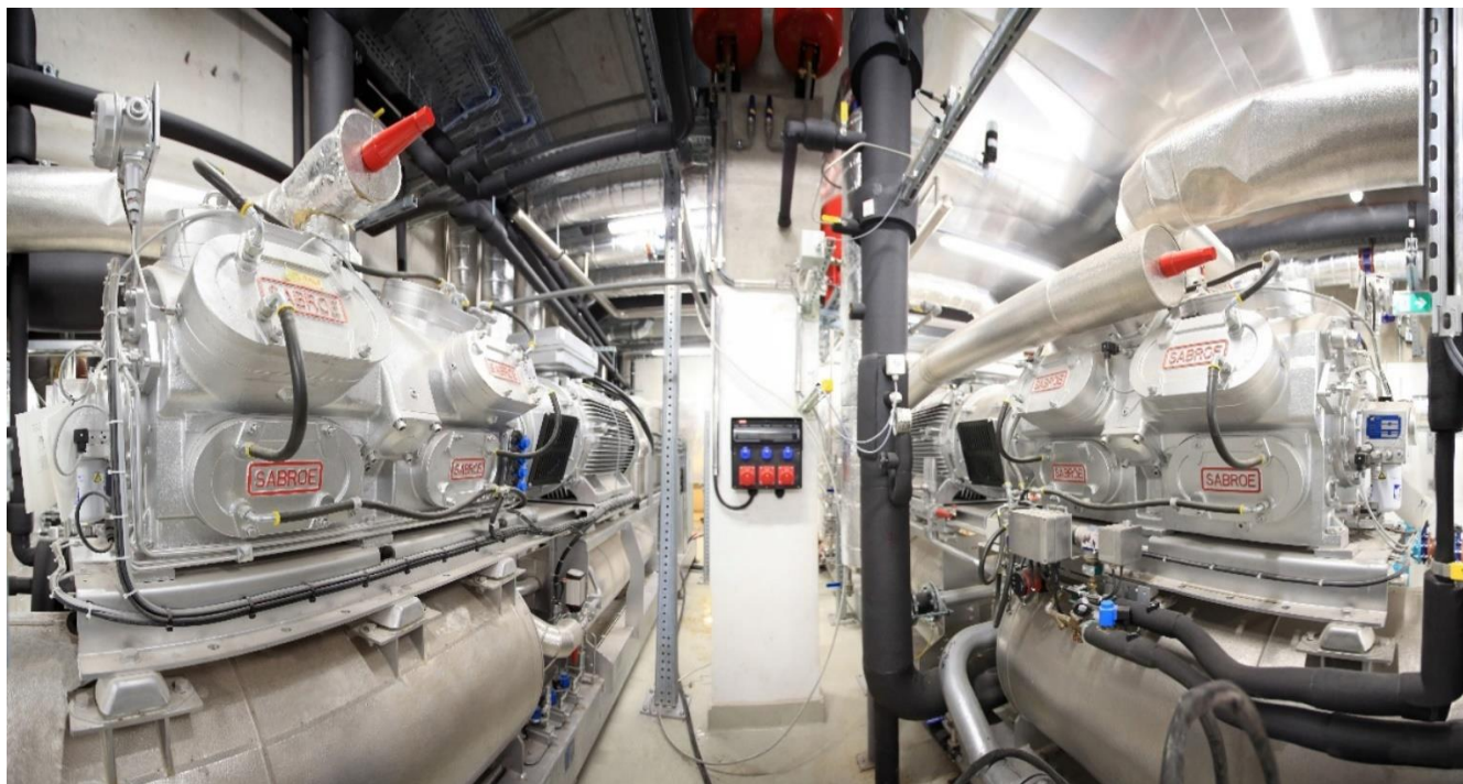
Figure 14: Heat pump system at spa Vienna (Source Klimafonds / Krobath)
