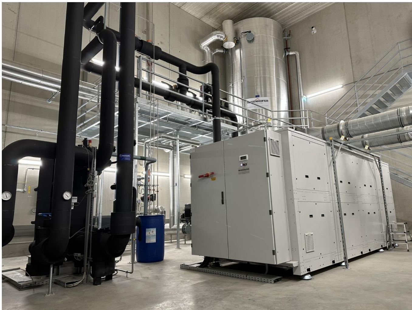
Figure 5: Heat pump within sector coupling concept in Gleisdorf (Source: Stadtwerke Gleisdorf)
