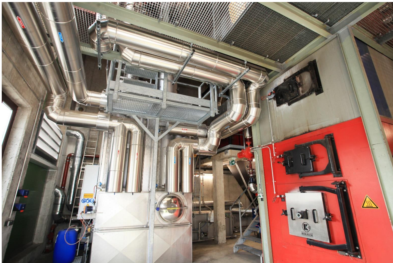
Figure 10: Flue gas condensation and biomass boiler in Saalfelden (Source Klimafonds / Krobath)
