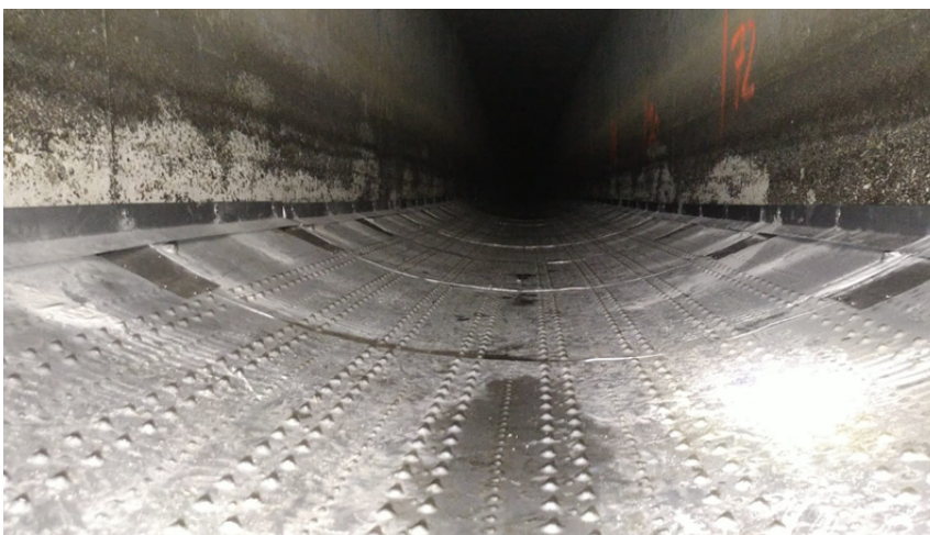
Figure 13: Custom made heat exchangers in the existing sewer (Source: Rabmer)
