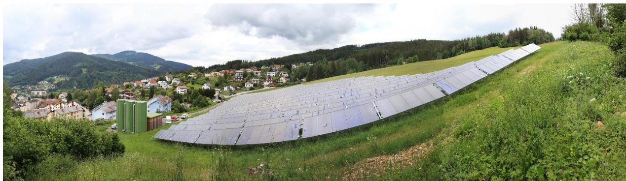
Figure 9: Solar plant in Mürzzuschlag (Source: Klimafonds / Krobath)
