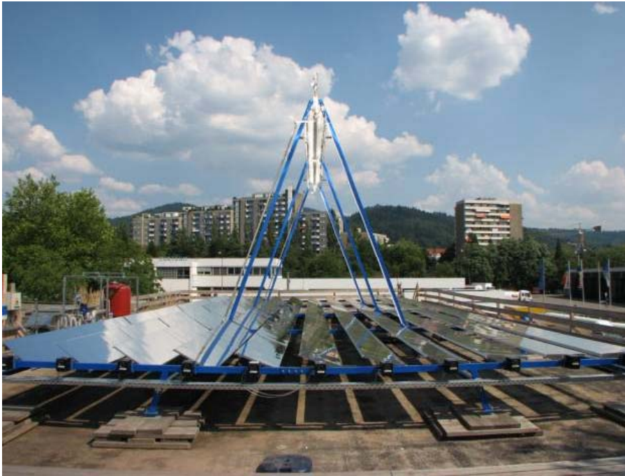
PSE Fresnel Collector, rooftop installation to power a NH 3 /H 2 O Absorption Chiller (Source: PSE, Germany)
