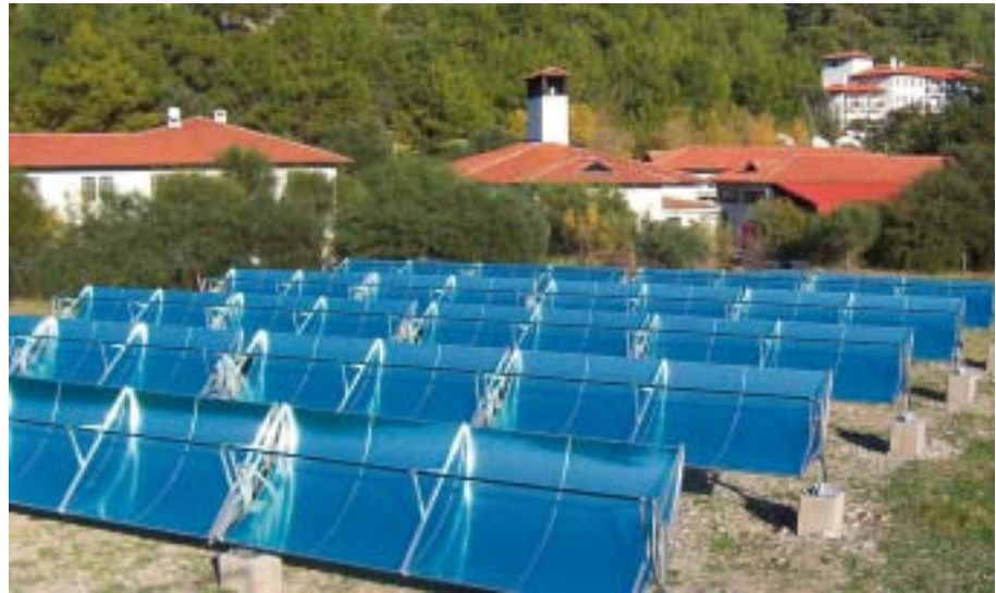
Fig. 16: 180 m 2 aperture area of parabolic trough collectors at a hotel in Turkey (picture source: SOLITEM, Germany)
