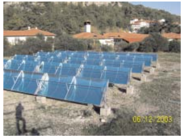
Prototype installation at Sarigerme Park Hotel in Dalaman, Turkey
