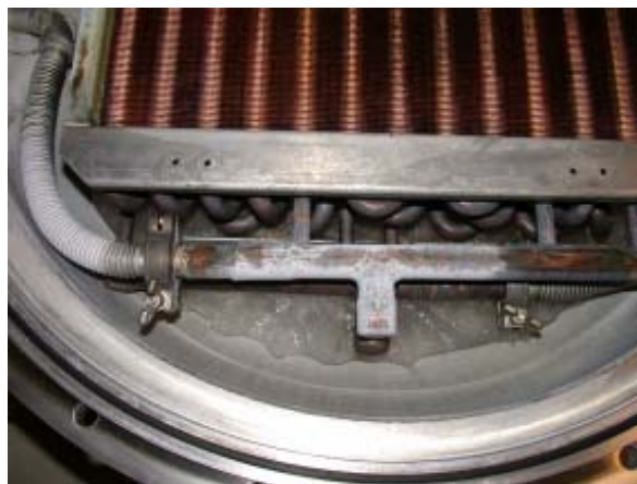
Fig. 34: View inside the evaporator area after freezing occurred
