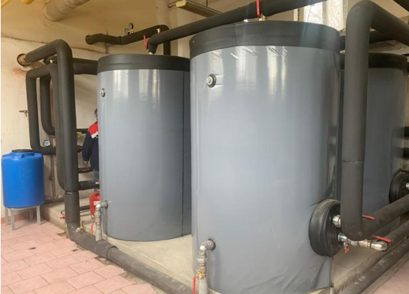
Newly installed air-to-water heat pump system in Lviv. Photos: Lvivteploenergo/City Institute Lviv
