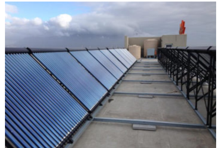
100 m 2 ST system with 20 m 3 hot water storage including heat pumps in Western Cape, South Africa
