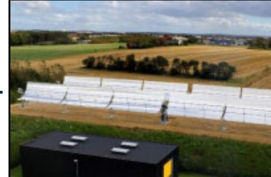
2011 CSP for district heating optimized for local conditions, Denmark
