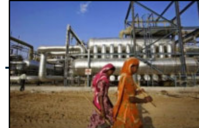
2013 50MWe and 25MWe steam generators, India
