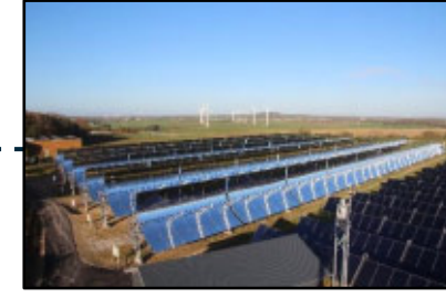
2015 CSP combined with flat panels for district heating, Denmark
