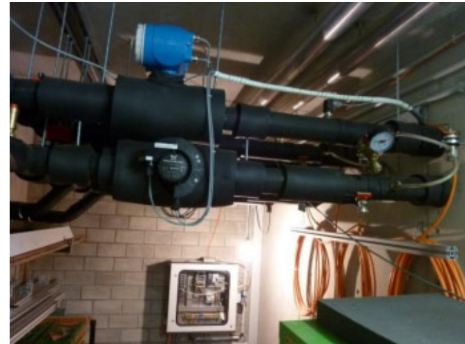
Peripheral equipment of the geothermal system
