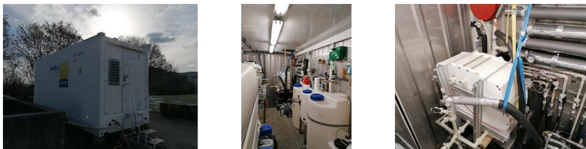
Figure 3: A membrane distillation unit installed in a container was installed for a two-month real operation at the wastewater treatment plant Gleisdorf (from right to left : container unit from outside, container from inside, membrane distillation module), (Source: AEE INTEC).
